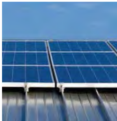
Roof mounted photovoltaic (PV) arrays
