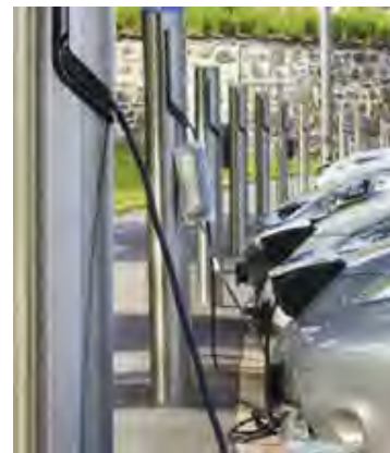
Electric car charging points
